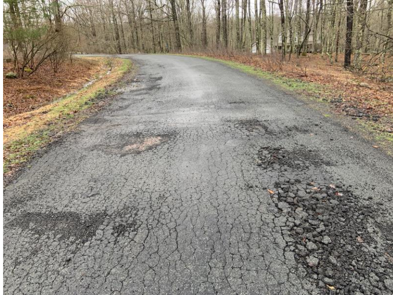
Figure 6 – Example of a deteriorated road surface that requires complete replacement
