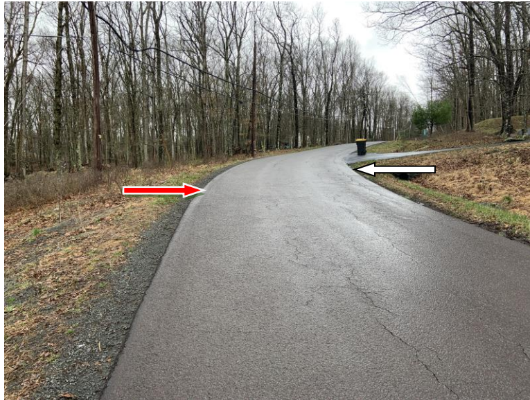
Figure 5 – Catamount improper cross slope
