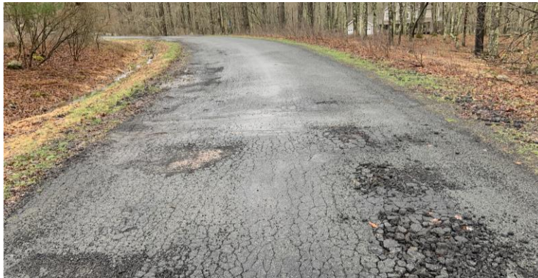
Figure 2a – Roadway deflection at culvert on Parkwood Drive
