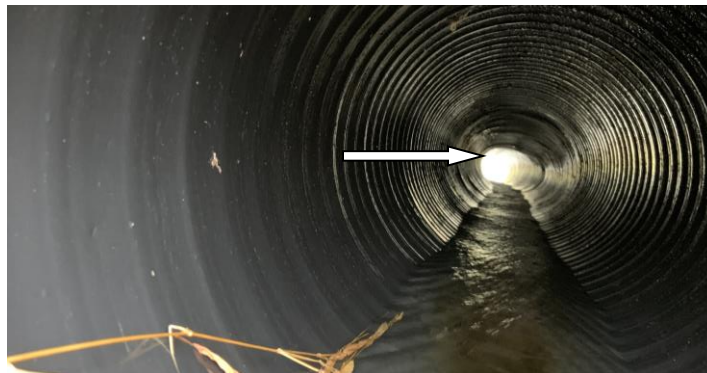
Figure 2b – Slight deflection of culvert on Parkwood Drive
